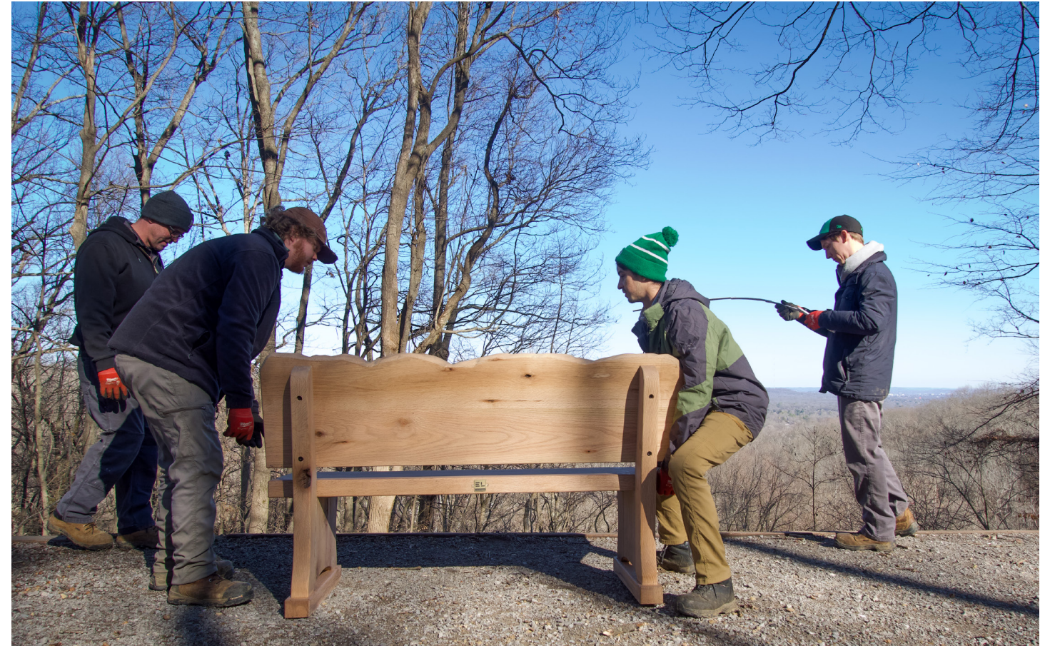
Above: Winter S.W.E.A.T. crew installs commemorative bench along the 11.2 mile loop in Percy Warner Park.
